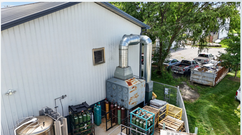
Air Filtration System
